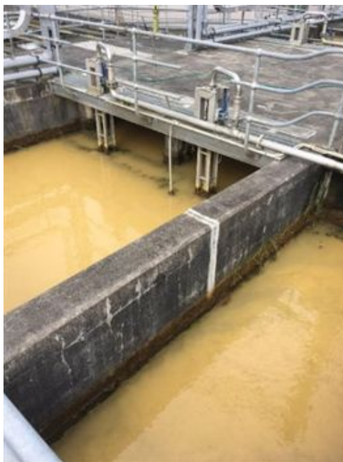
Incoming water 9 March 2017, Ardmore WTP
